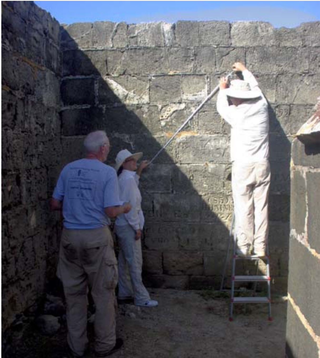
Figure 26. Rod, Rosanne and Mark measuring control points needed for the rectification of digital photos. Graffiti on the enclosure wall of the Powder House is being recorded and drawn using this technique. (04jv2111)
