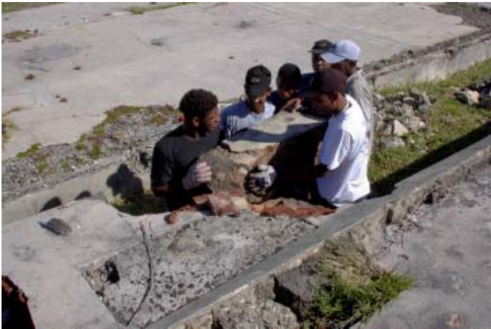
Figure 24. The workmen uniting efforts to put back a large basalt block dislodged from the settling tank of the Cistern. (04jv0905)
