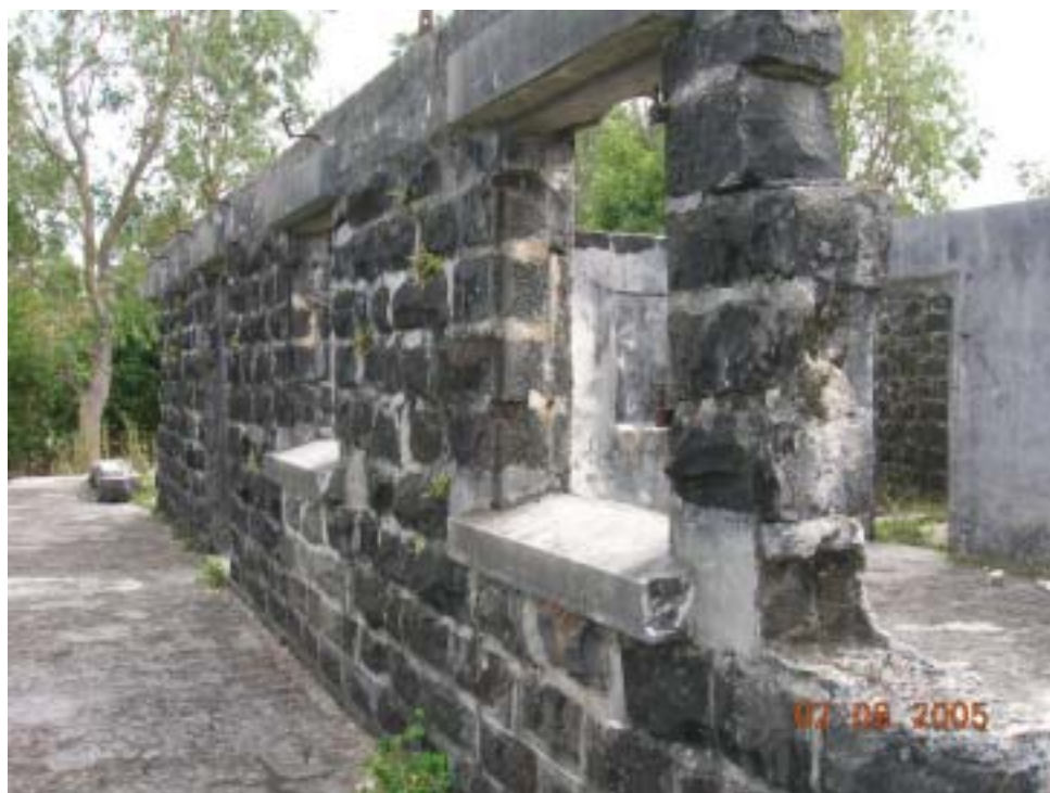
Figure 31. Roofless masonry building. (md05nn0148)
