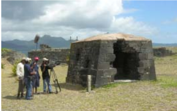
Figure 29. The Hot Shot Furnace needs urgent attention if further collapse of the roof is to be prevented. (mp06nc0802)
