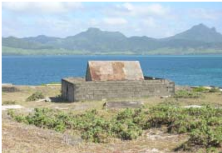
Figure 30. The Powder House continues to suffer from fires lit very near its fragile walls. (mp06nc0103)
